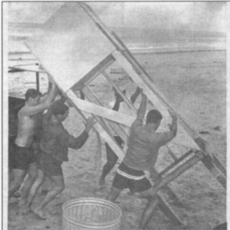
HEAVY SUMMER BEACH traffic will soon start and the area lifeguard captains are preparing, training, and increasing their staff. At the Del Mar Beach, Capt. Gardner Stevens and five new lifeguards put up a temporary tower at the 20th Street beach. Del Mar now has a tower at 17th, 20th, and 25th Streets to increase surveillance of swimmers.
